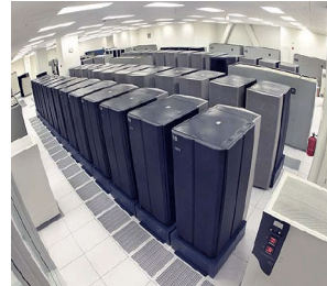
(D) Dyna-Vision™ Server in hosted facility
